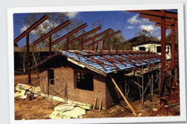
Image supplied by the Townsville Cyclone Testing Station
